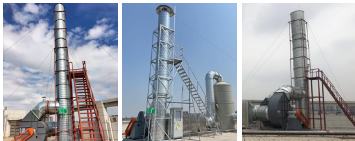
Waste Gas Disposal Facilities
