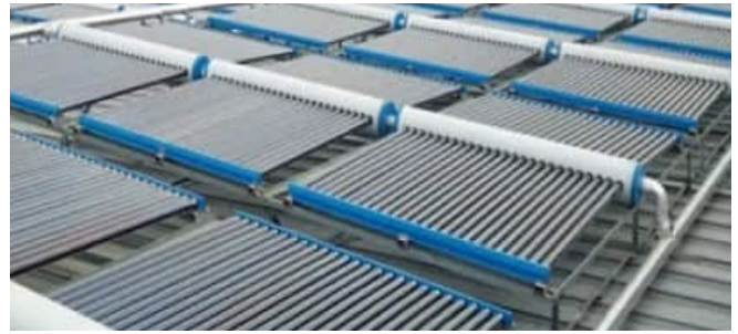
Nanchang Solar Water Heating System
